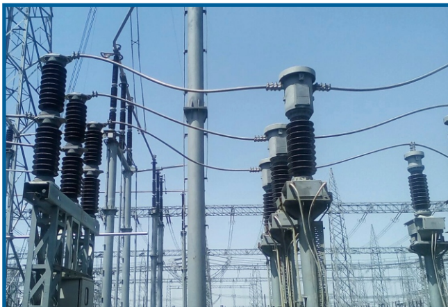
Substation without IEP Products
