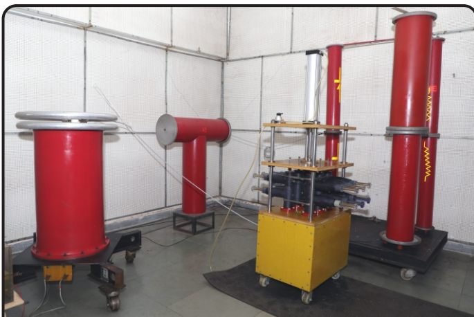
High Voltage Test Lab
