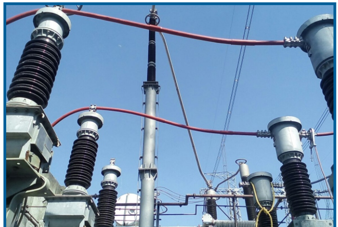
Substation installed with IEP Products
