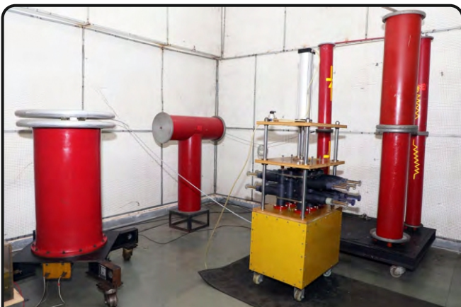
High Voltage Test Lab
